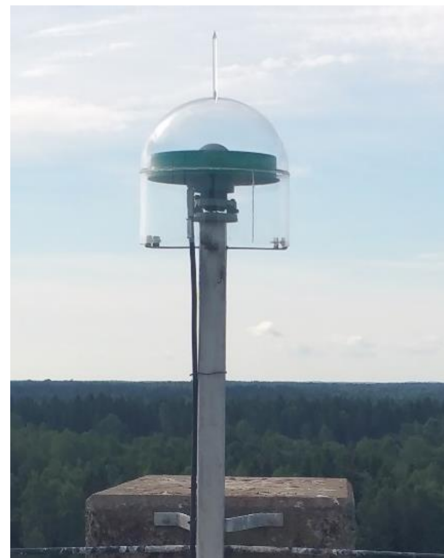
Figure 2: The OSOP radome installed at the SWEPOS station Trollhättan.
